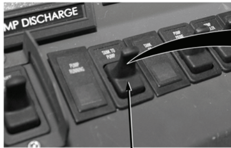
TANK TO PUMP SWITCH
