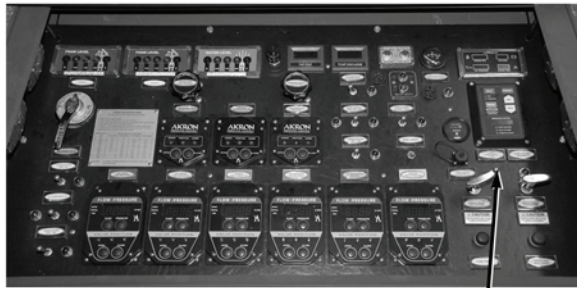
START PUMP ENGINE STOP SWITCH
