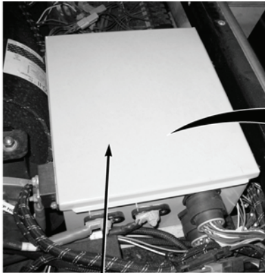
PUMP HOUSE POWER DISTRIBUTION
