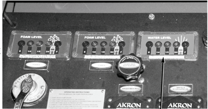
PUMP OPERATOR'S PANEL WATER LEVEL GAUGE
