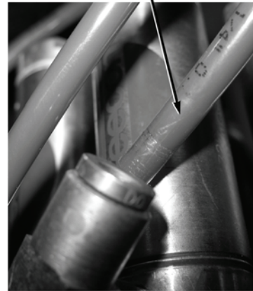
AIR LINE AT ROOF TURRET FOAM B MULTI-METERING VALVE CYLINDER
