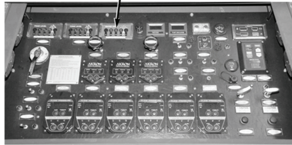
PUMP OPERATOR'S PANEL WATER LEVEL GAUGE
