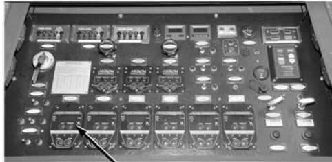
NO. 1 DRIVER SIDE DISCHARGE VALVE CONTROL
