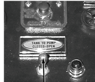
TANK TO PUMP SWITCH
