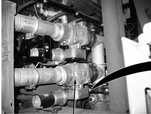
NO. 4 PASSENGER SIDE DISCHARGE VALVE
