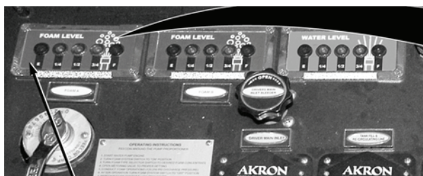
PUMP OPERATOR'S PANEL FOAM A LEVEL GAUGE
