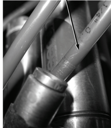
AIR LINE AT BUMPER TURRET FOAM A MULTI-METERING VALVE CYLINDER
