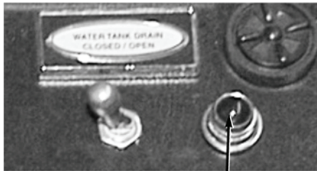
WATER TANK DRAIN INDICATOR
