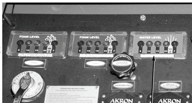
PUMP OPERATOR'S PANEL WATER LEVEL GAUGE
