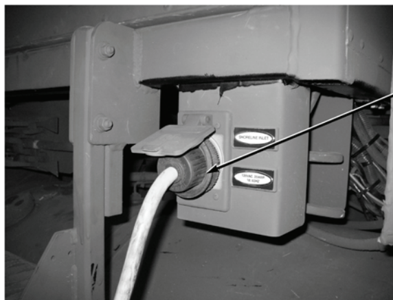
SHORELINE INLET RECEPTACLE WITH POWER CORD CONNECTED
