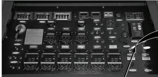
START PUMP ENGINE STOP SWITCH
