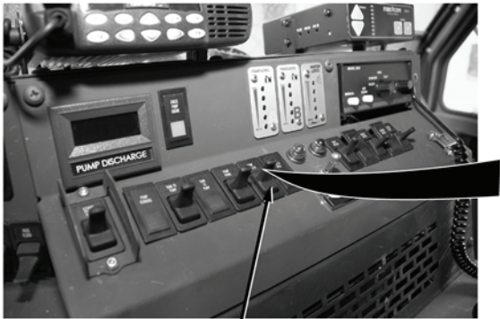
PUMP COOLER SWITCH
