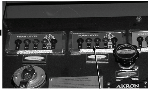
PUMP OPERATOR PANEL FOAM B LEVEL GAUGE
