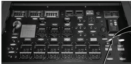
START PUMP ENGINE STOP SWITCH
